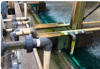
BEFORE EasyWater Treatment – Excessive algae present and the water is turbid
