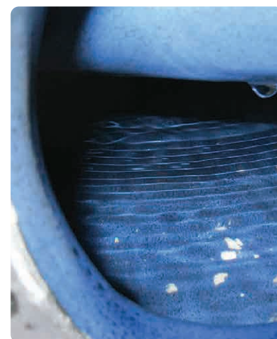
AFTER: 4 Months — Water Heater with EasyWater Treatment
