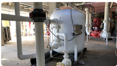
Sand Filters Prior to Installing EasyWater CTF Systems
