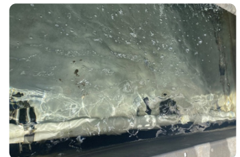
AFTER TWO WEEKS - Algae in the cooling tower sump basin was eliminated in two weeks
