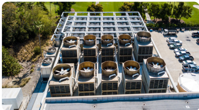
12-Cell, 8,000 ton cooling tower system
