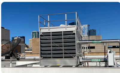
BAC cooling tower on the roof
