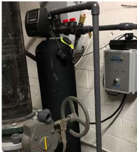
EasyWater Series C System: Model CLC-1000 Installation at CocoWalk
