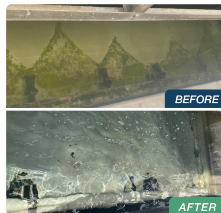
Algae in the cooling tower sump basin reduced after two weeks
