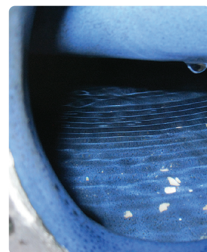
AFTER: 4 Months — Water Heater with EasyWater Treatment
